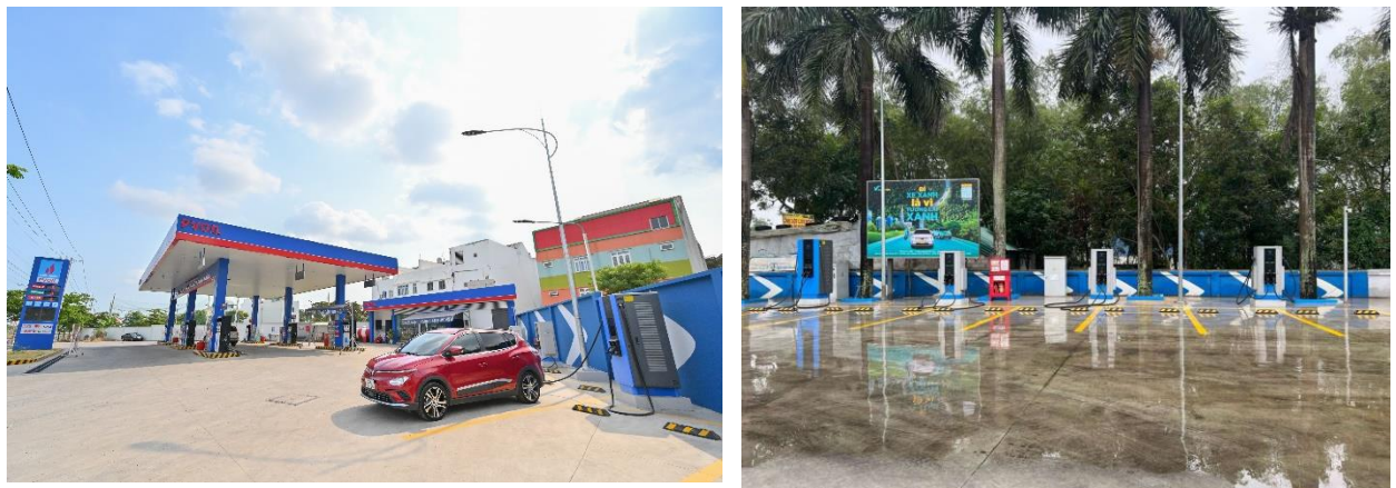
Some pictures of Vinfast's electric vehicle charging station at PVOIL's petrol station
